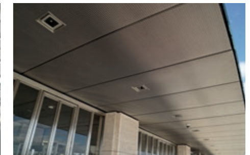
Ceiling made from framed mesh elements. Krasnodar, Stadium, Russia, EGLA-MONO 5031.
