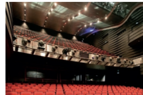
Curved ceilings. Bielefeld Town Theatre, Germany, MULTI-BARRETTE 8123.
