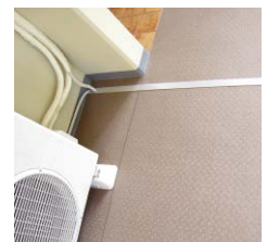
Air Conditioner Drain Pipe
