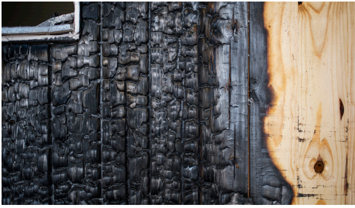
Charring is the result of flame and heat that provides the CLT's fire resistance. Courtesy photo by Erika Edwards.
