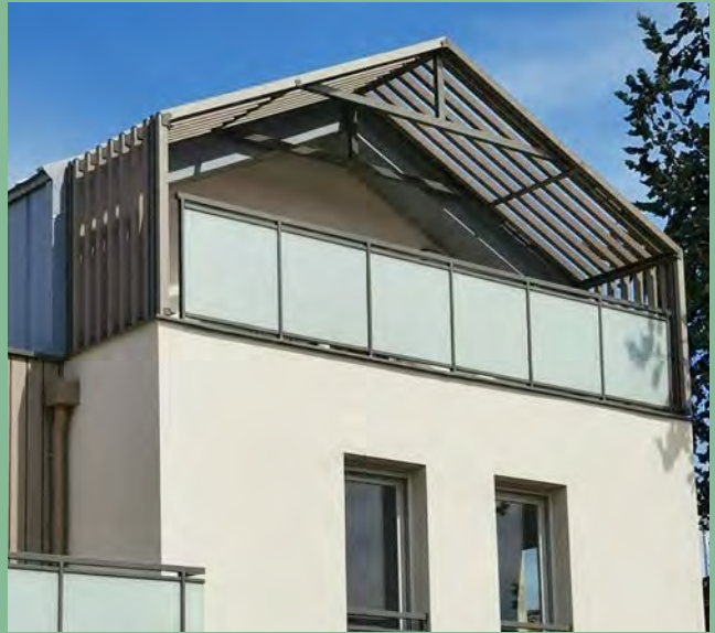
SPACE 6 - Farbton Sand • Architekt: Anne Terrier / Ann'T Architecture
