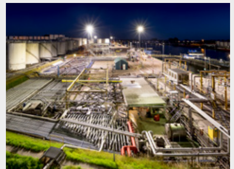
Tank storage Standic B.V. | Dordrecht | Netherlands
