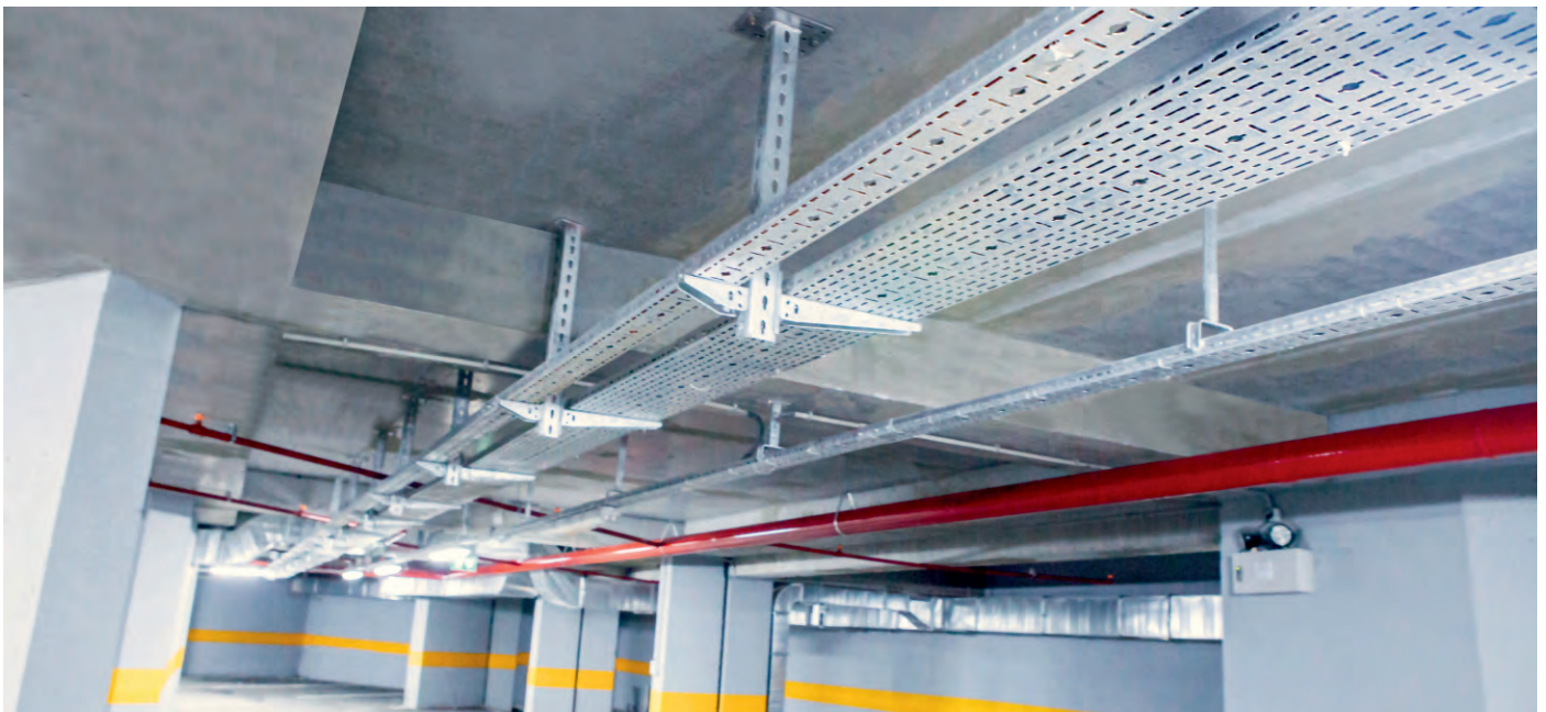
Cable tray application
