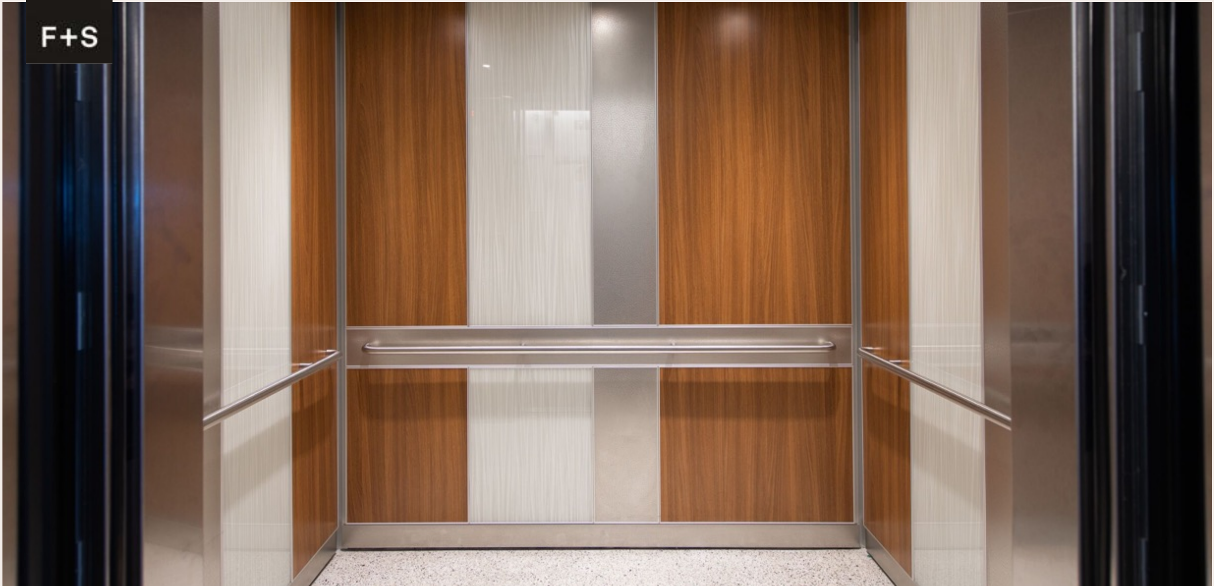
LEVELe Elevator Interior, ViviGraphix Graphica glass, Stainless Steel. Round Handrails. Elevator Ceiling | UCHealth Highlands Ranch Hospital
