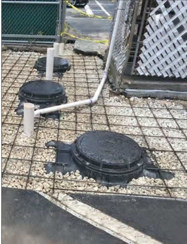
Two BIG-1150 Grease Interceptors installed in a Miami, FL restaurant
