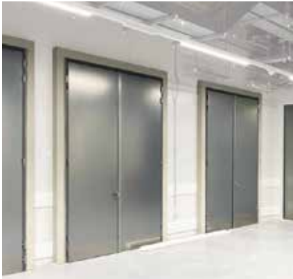
Datacenter / IT room
