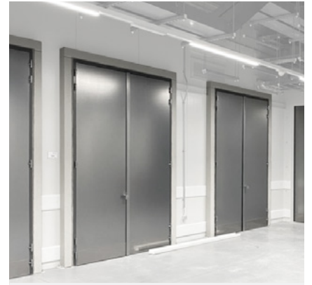
Datacenter / IT room
