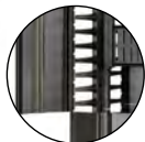
Side cable openings align with U marks on the rack
