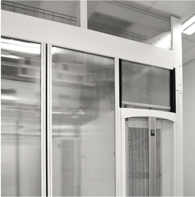
UF Health Shands utilized CPI’s custom HAC Solution to maintain cooling, while accommodating storage solutions of various heights, widths and depths.
