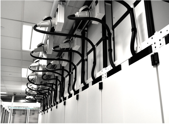
CPI manufactured custom cable openings into the cabinets to fit UF Health Shands' unique design.
