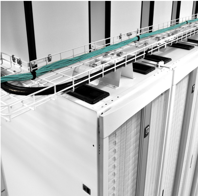
CPI’s Wire Mesh Cable Tray provides point-to-point pathways for the network cabling in the data center.
