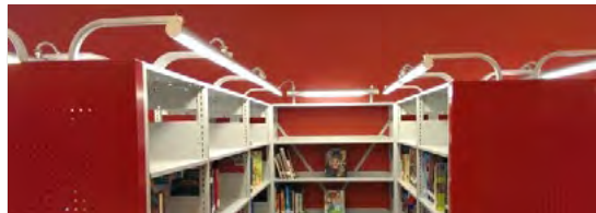
LED AISLE LIGHTING
