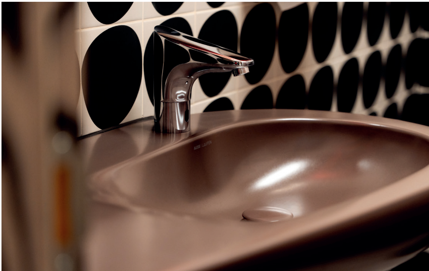
Brewery Cēsu alus – ILBAGNOALESSI washbasin Cēsis/Latvia Architecture: Anete Antonevica Interior and Zane Apsīte
