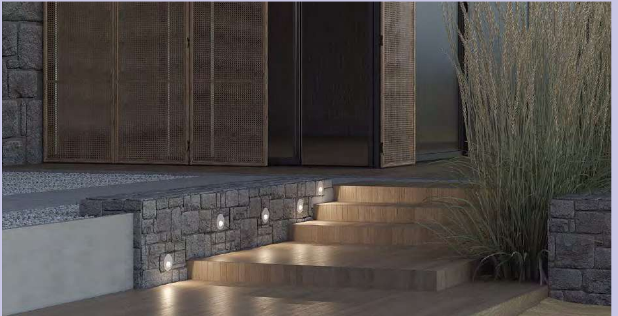
Bil Staircase Lighting
