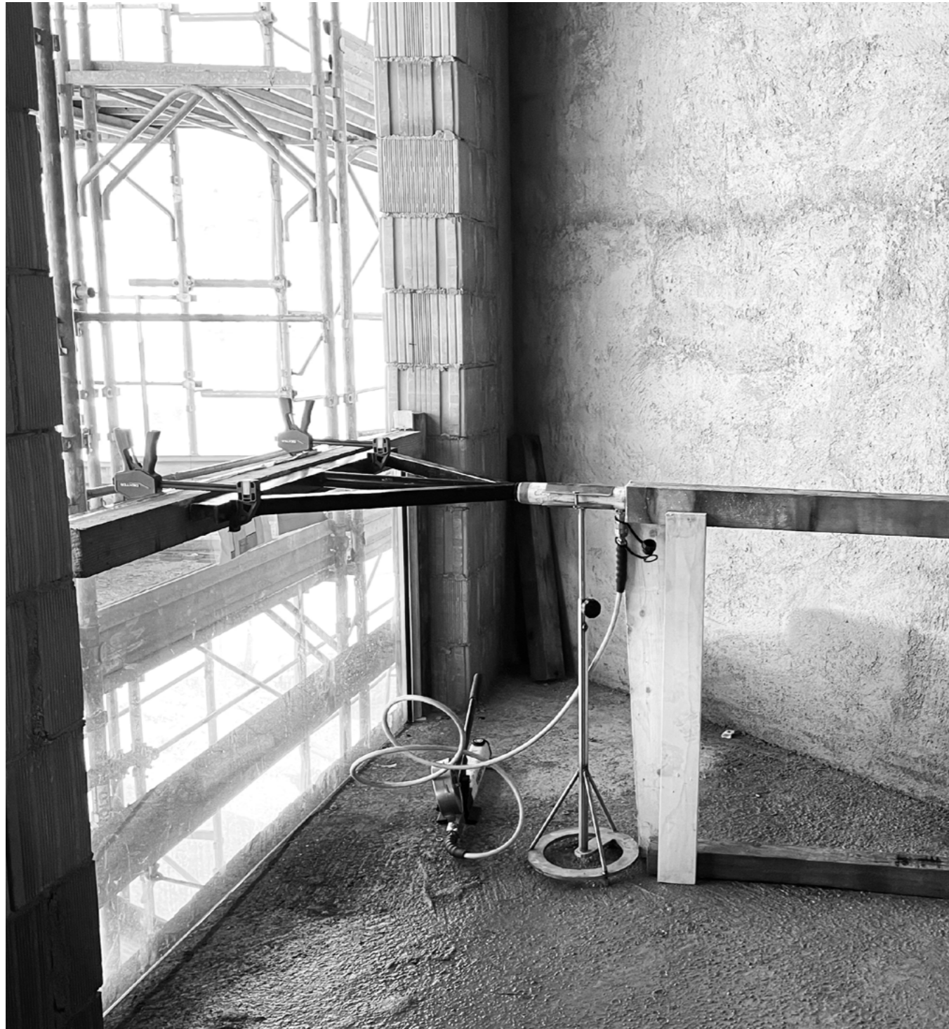
Example of an on-site test with static load test up to 300 kg/m with a 10+10 glass 250 cm wide and 110 cm high, with totally positive results
