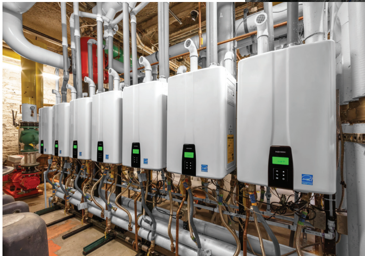
14 high-efficiency NPE-2 tankless water heaters supply endless hot water to the hotel's guests and facilities.
