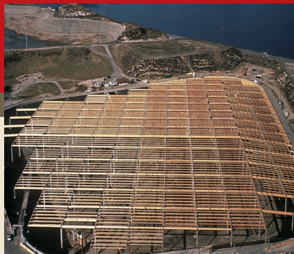
Red-H™ trusses—60 feet long and up to 6 feet deep—form the structural backbone of this 12-acre reservoir cover, which was specially engineered to withstand both vertical and horizontal loads.
